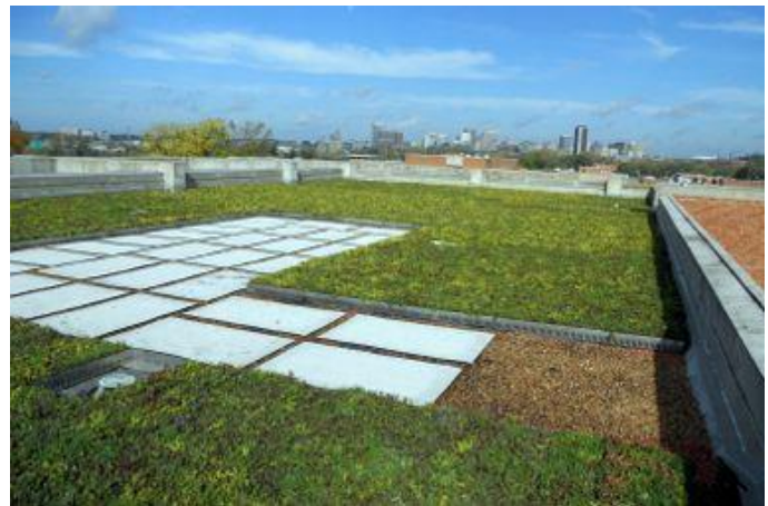
Waste Water Treatment Plant Effluent Filtration Building, Richmond, Virginia
